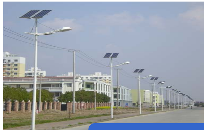
郊区太阳能路灯 Solar-energy Road Lamp in Suburb
